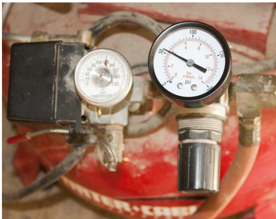
Air compressor set up. Supply tank pressure on the left gauge, output pressure controlled by knob below on the right.
